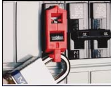
Circuit Breaker Lockouts
